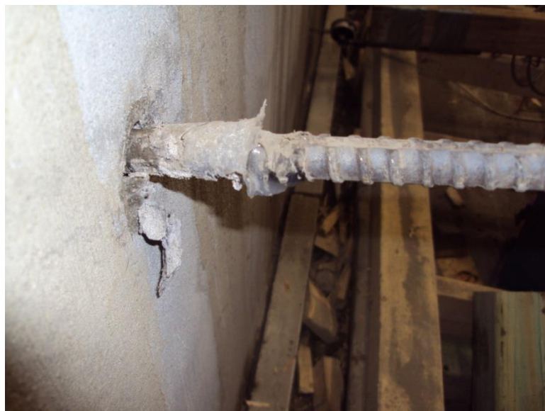
Figure 3.34: Pullout failure of rebar in CLSM abutment.
